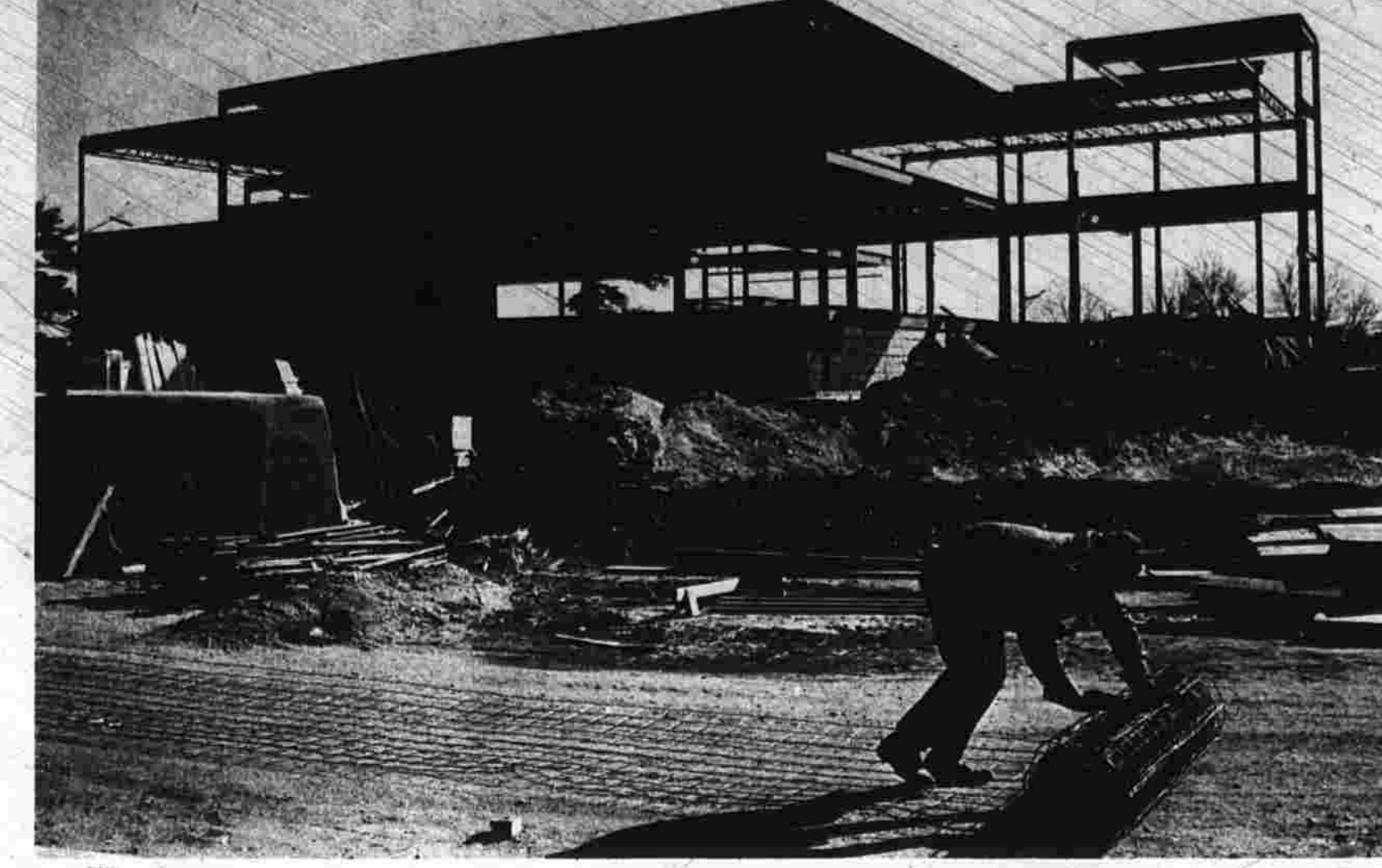
Work rolls on at the construction site of the new South Windsor town hall behind the Peapack Community Church at Sullivan Ave. and Ellington Rd. The A. F. Pease Construction Co. of Hartford is "on schedule," according to Mrs. Alice Green of the Public Building Commission. It is expected to receive crowd conditions at the old town hall on Main St. when it opens early this fall. Building cost of the 21,000 square foot structure is $414,056. (Herald photo by PhotoVision)
